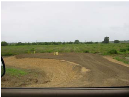
Potable water system access
